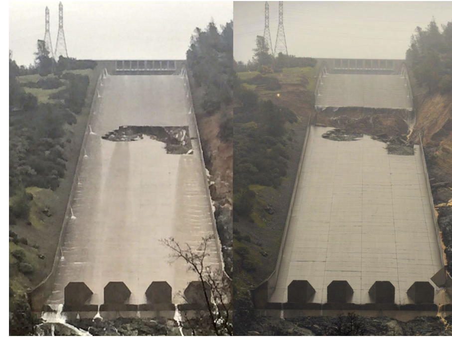
Source: https://geotechpedia.com/News/Show/953/Oroville -Dam-Spillway -Failure
