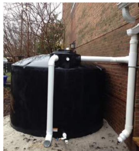
Figure 22 – Example cistern application
