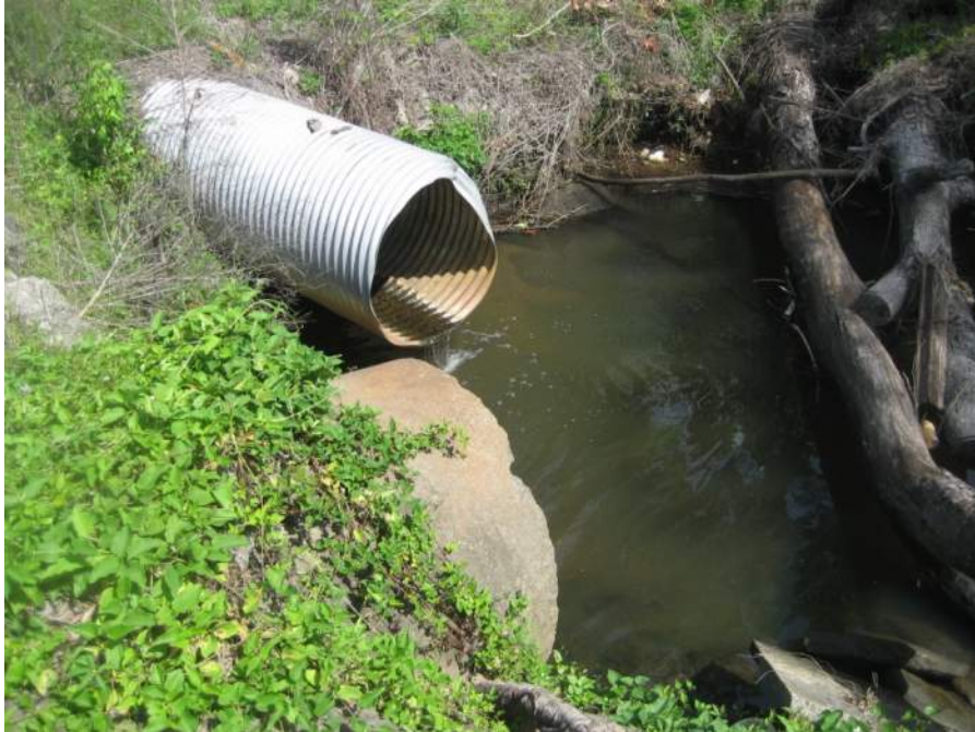
Figure 11 – Example of untreated stormwater entering Goose Creek tributary along Murray Avenue
