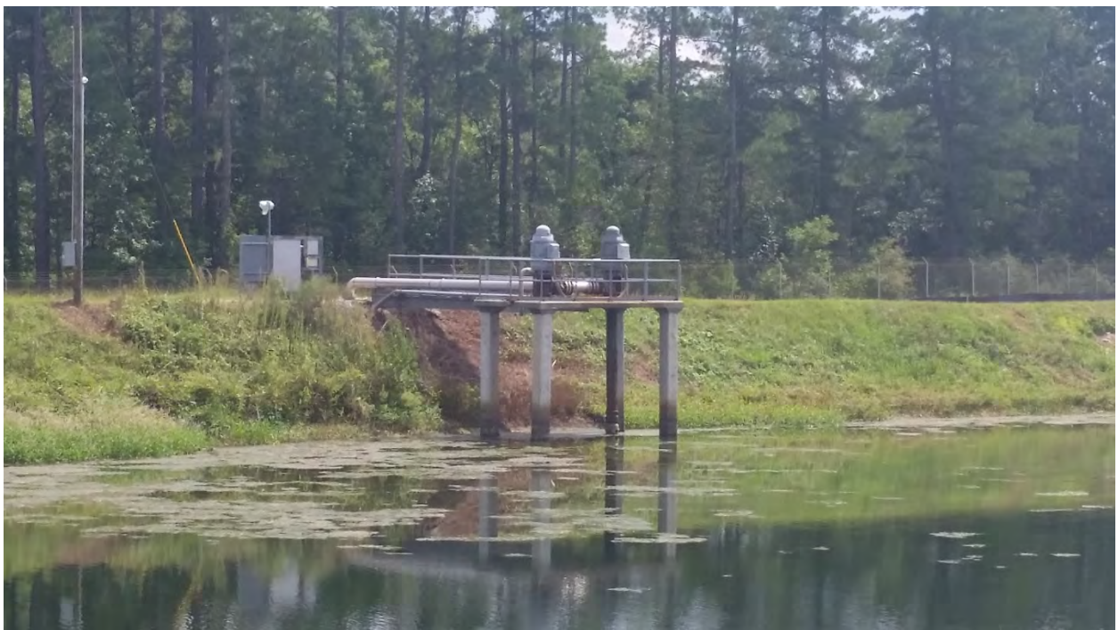
Figure 16 - Spray Pond NW Pump Station
