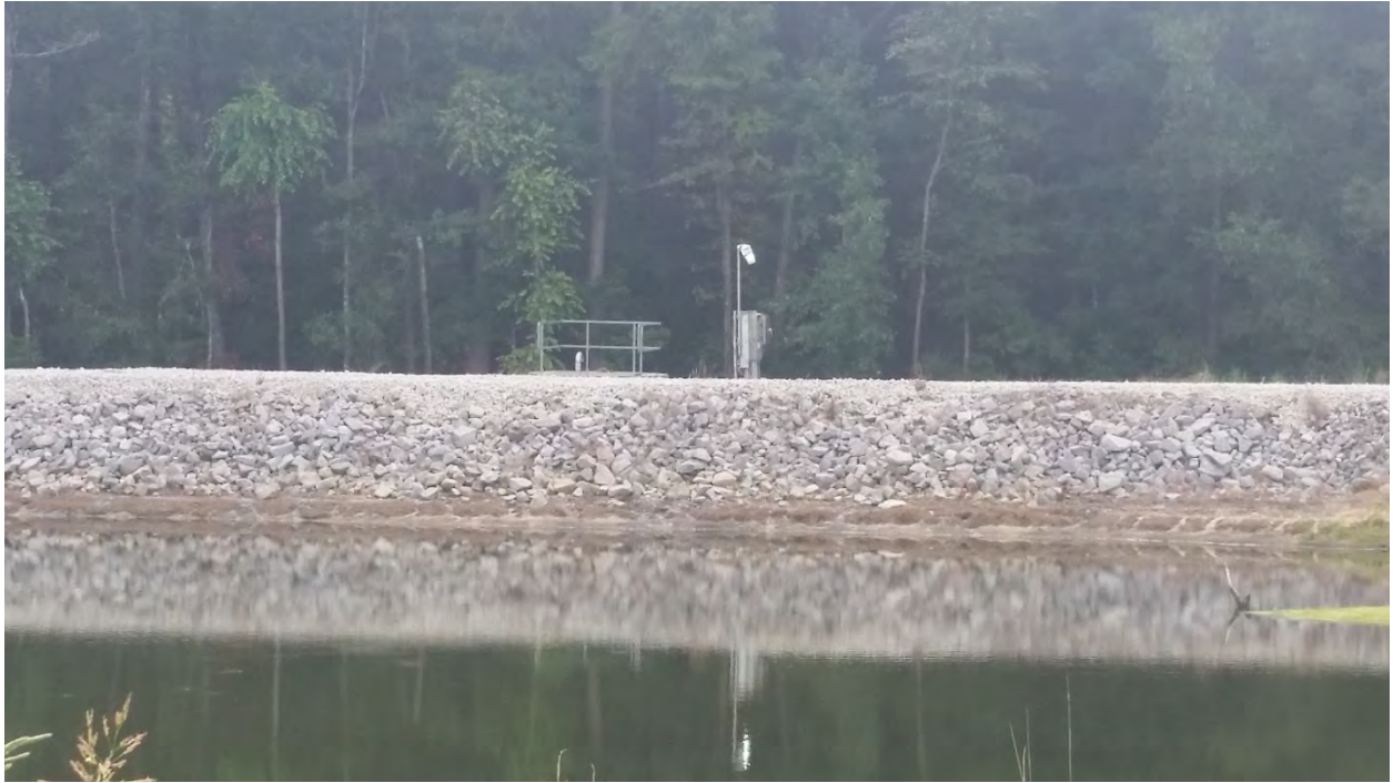
Figure 3 - Settling Pond #2 Pump Station
