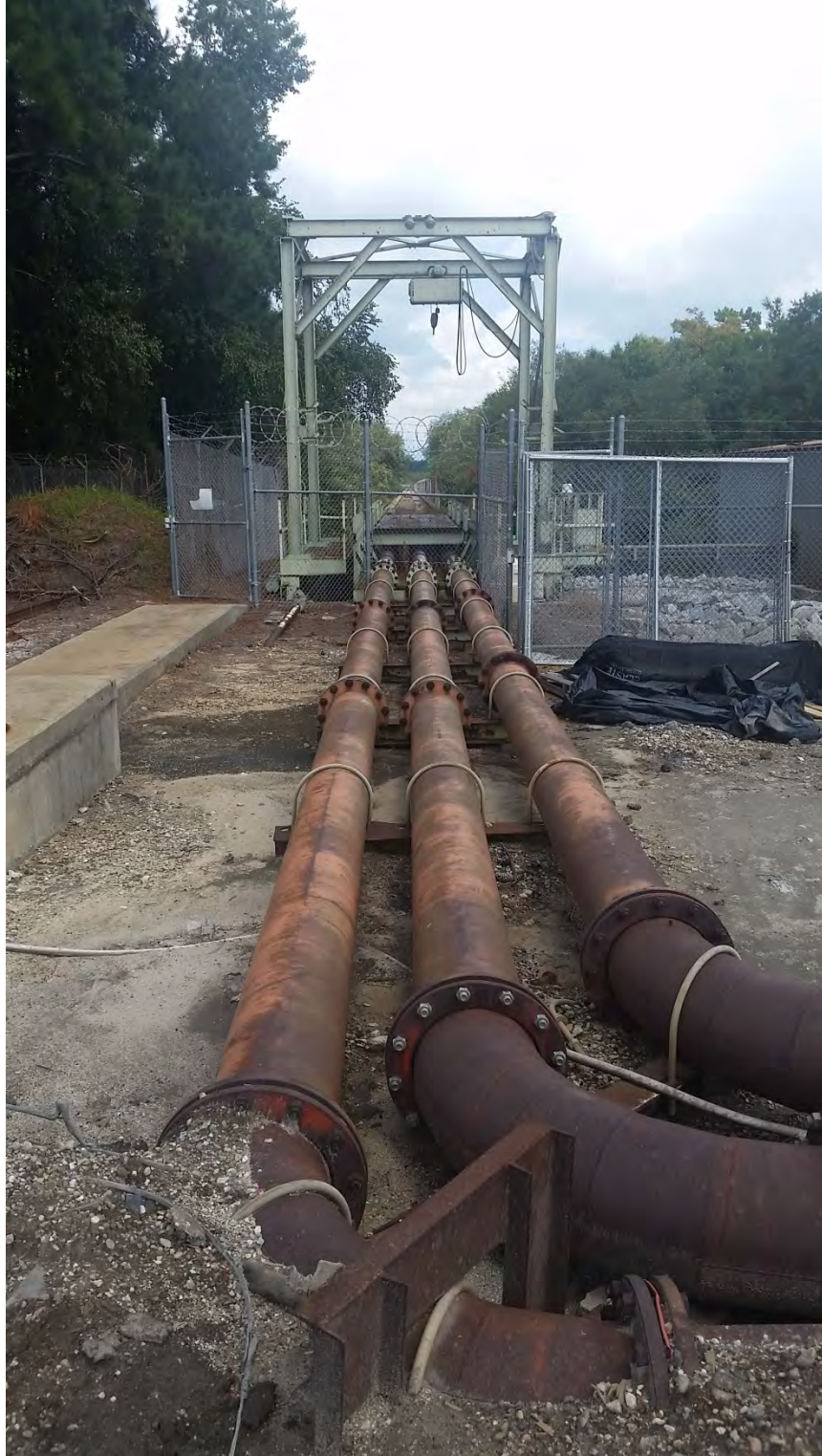
Figure 17 - Piping & Bridge System (to AP2 & Outfall 006)
